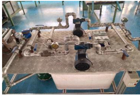
Fig. 1. Pump Installation with a Manual Control System
