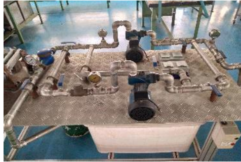
Fig. 1. Pump Installation with a Manual Control System
